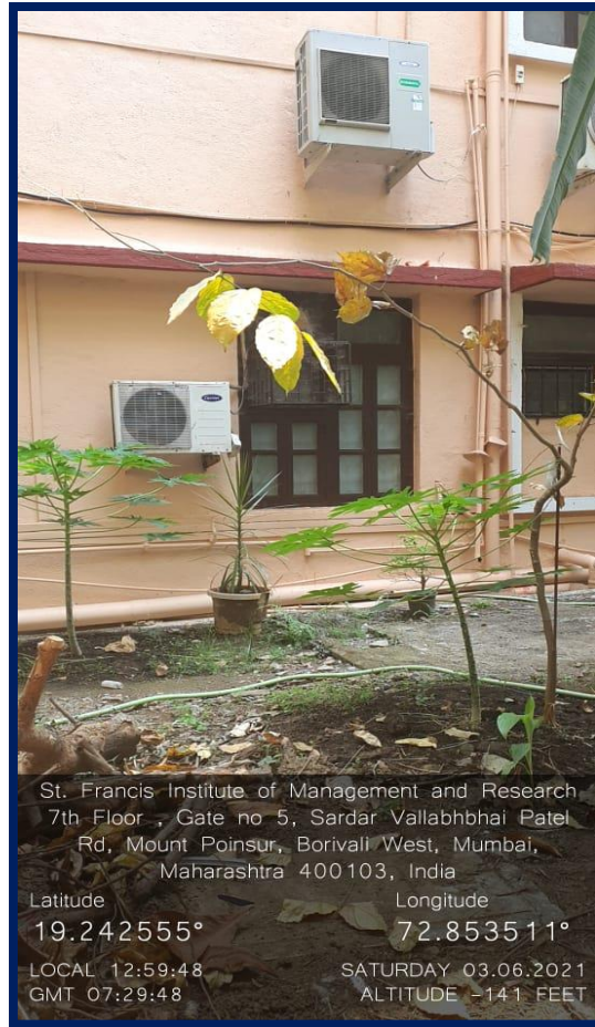
Brought down by vertical & Horizontal Pipes
