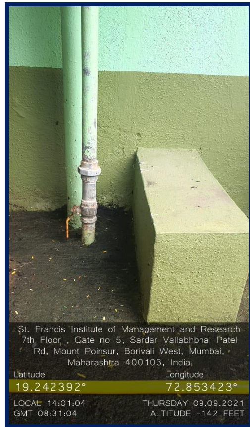
Pipeline from bore well tank to Hostel
